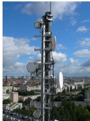
Microwave backhaul site
